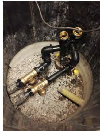
Figure 3.2: Top of the coaxial borehole
